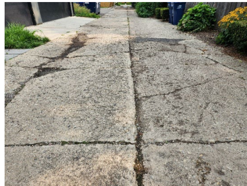
Example of a Serious Concrete Alley
