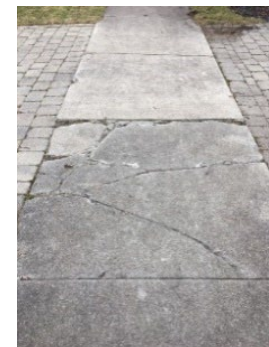
Cracking with Displacement
