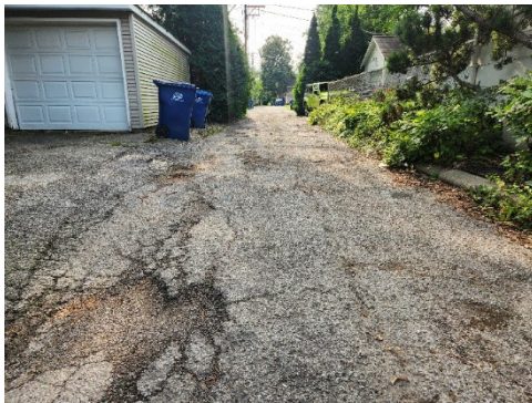
Example of a Serious Asphalt Alley
