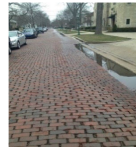
Localized Edge Settlement
