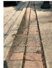
Brick settlement behind curb
